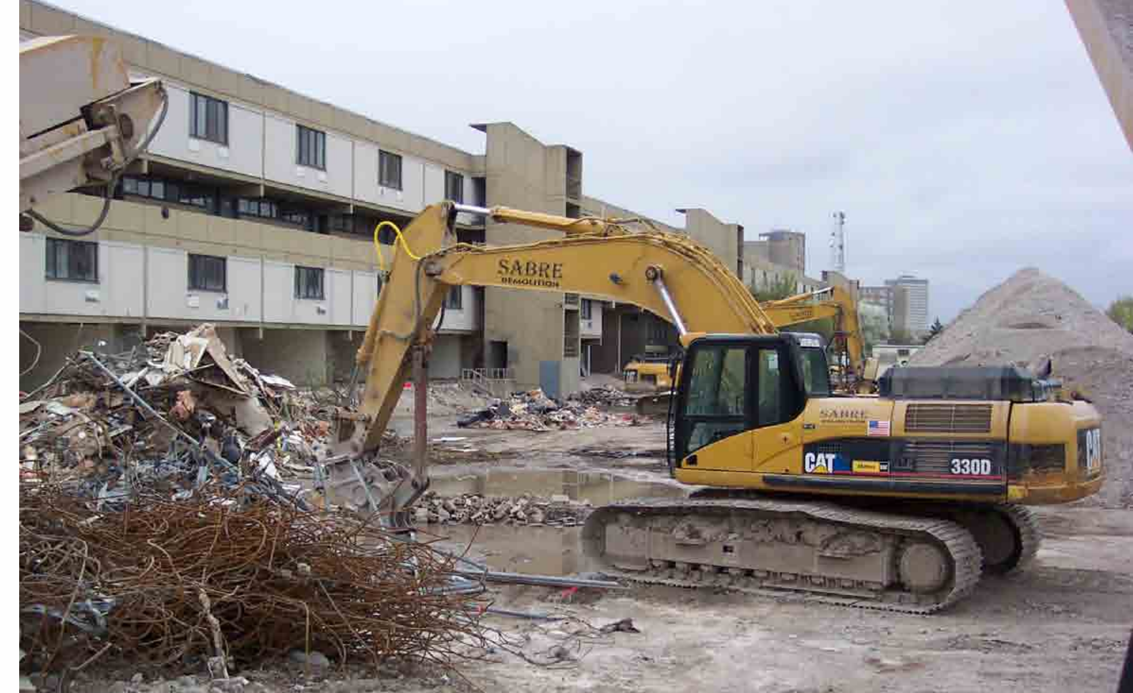
Former apartment buildings during demolition with recycled concrete pile to the right.
